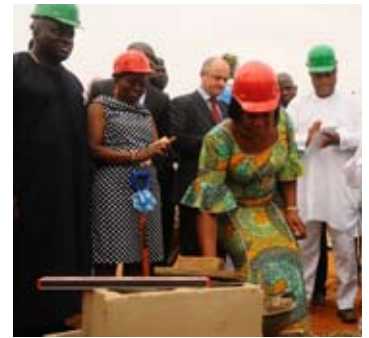
Nigeria's Minister of Aviation, Mrs Fidelia Njeze lays the foundation blocks for the Lagos Hilton Hotel.
